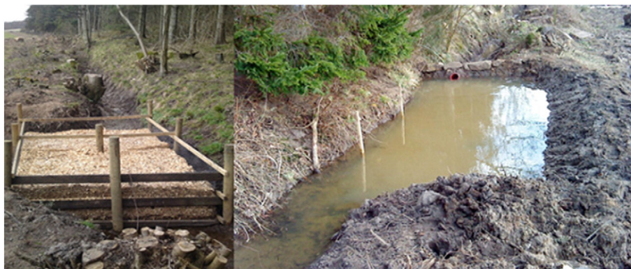
Fig. 6. Wood chip filter (left) and a sediment trap (right) placed in ditch upstream of RAF 12.
