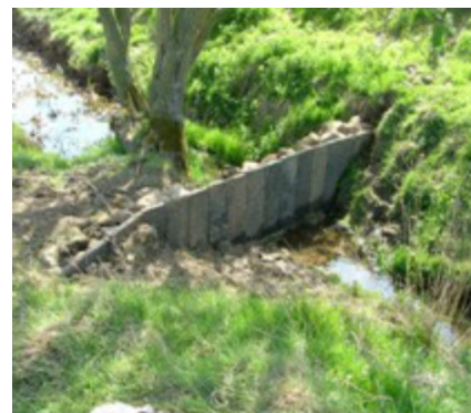
Figure 10 – Online barrier in small farm ditch
