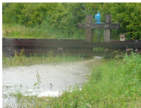
Figure 17 – Outlet Sluice from field pond
